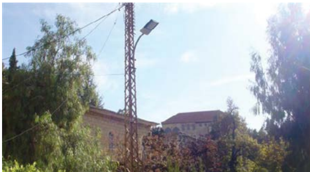
Figure 9-20 PV Street lighting in Mokhtara Municipality, Chouf Photo Credit: CEDRO Project
