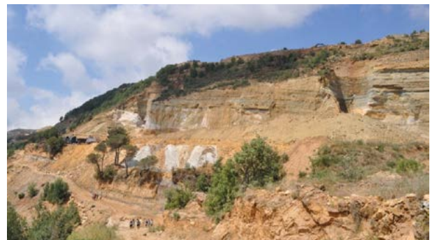
Figure 6-10 Excavation for Construction Leading to Loss of Topsoil and Erosion in Hrajel, Keserwan Source: Yazigi Atelier, 2014
